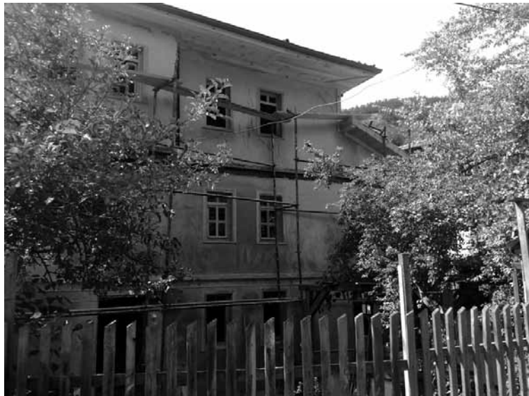
Figure 6. A traditional house of Mudurnu undergoing restoration works with funding from the Ministry of Culture and Tourism (photo: E. Yıldırım, 2009)
