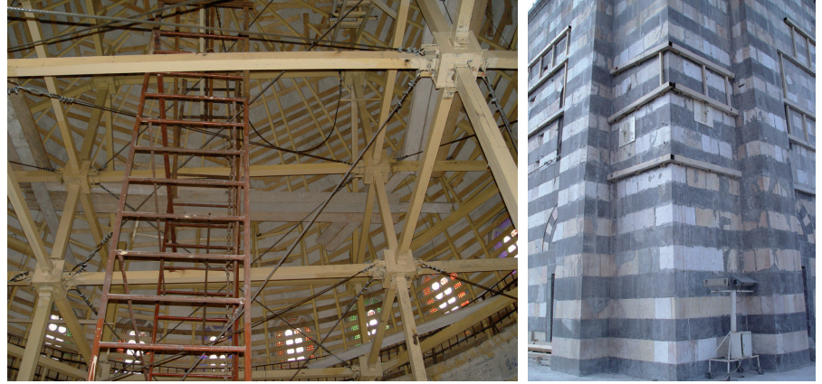
Figure 30. a) Steel framework system supporting the dome of Süleymaniye Mosque, b) Metal supports at the southern (kibla) wall of the Mosque, 2005.
