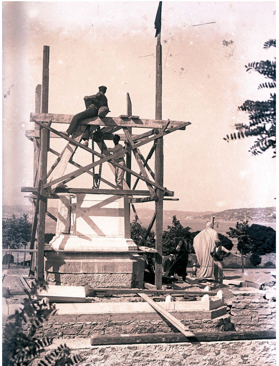
Figure 1. Sarayburnu Atatürk Monument under construction, September, 1926 (Suna and İnan Kırâç Foundation, Istanbul Research Institute Archive).
